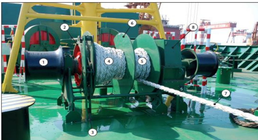
Electric mooring winch with split-type drum on the Forecastle Deck
